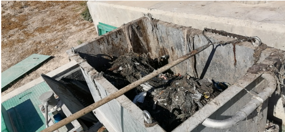
Photo (6): container of screen 50 mm in Jericho WWTP
