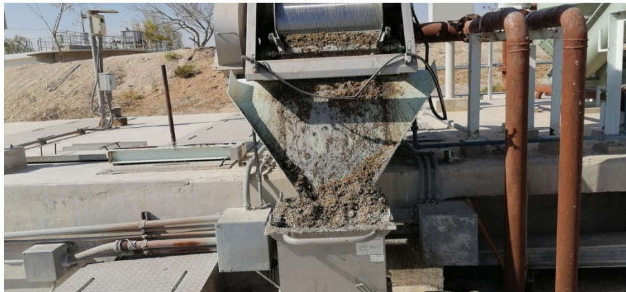
Photo (10): container of scum removal in Jericho WWTP
