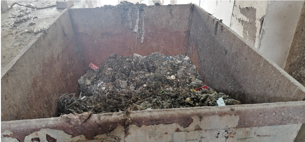
Photo (4): container of screen 6 mm in Al Tira WWTP
