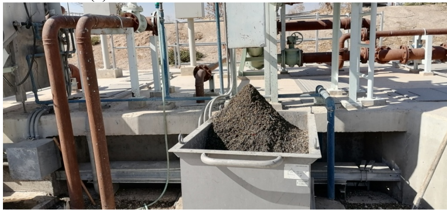
Photo (8): container of grit removal in Jericho WWTP
