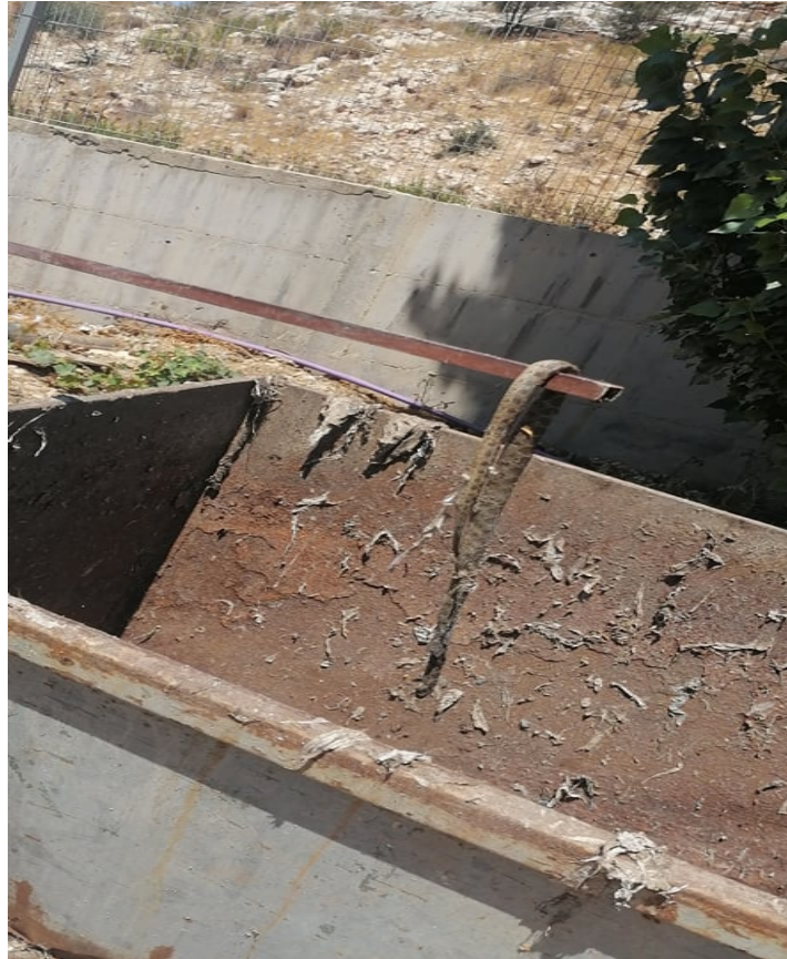
Figure 8| Snake in screen 50 mm in Al-Tira WWTP
