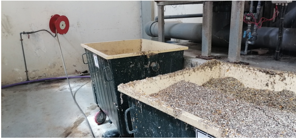
Photo (5): container of screen 2 mm in Al Tira WWTP
