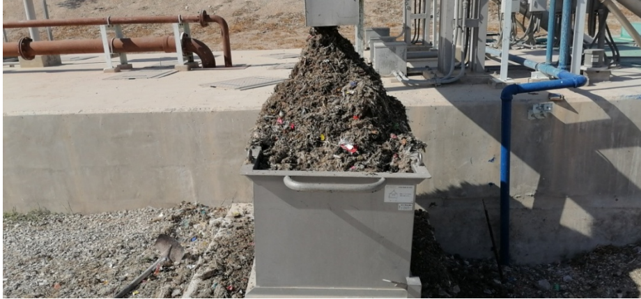
Photo (7): container of screen 20 mm in Jericho WWTP
