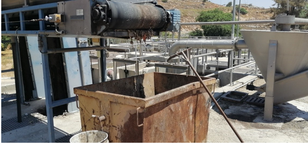
Photo (1): container of screen 50 mm in Al Bireh WWTP
