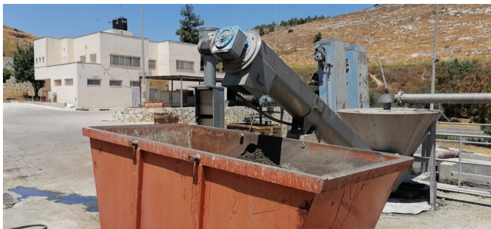
Photo (3): container of grit removal in Al Bireh WWTP
